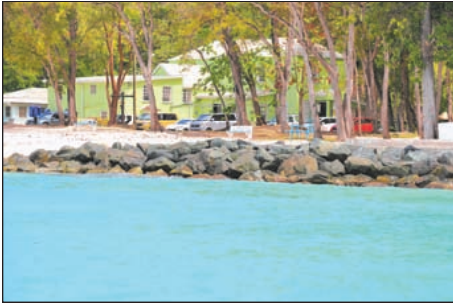
Some of the groynes installed at Folkestone Beach in Barbados. IPS/Desmond Brown
