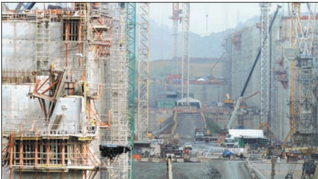
Cranes tower over the construction site of Panama Canal's Pacific expansion project in Cocoli, on the outskirts of Panama City, Friday, Aug. 8, 2014. August 15, marks the 100th anniversary of the Panama Canal construction, as it undergoes the biggest expansion project since it opened in 1914, which will allow larger Post-Panamax ships to cross the canal.
