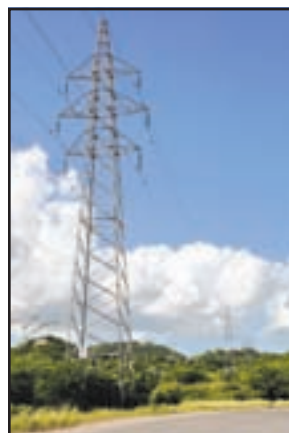
Power lines in Antigua. The Caribbean country is taking steps to achieve energy security through clean technologies.
