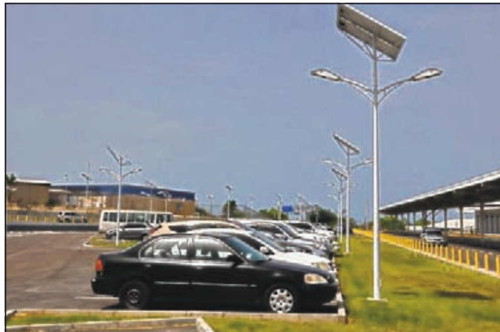
The light-emitting diode (LED) is one of today's most energy-efficient and rapidly-developing lighting technologies. Under the Japan-Caribbean Climate Change Partnership (J-CCCP) project, the community of Bartica is set to benefit from the installation of energy efficient as well as LED street lighting.
