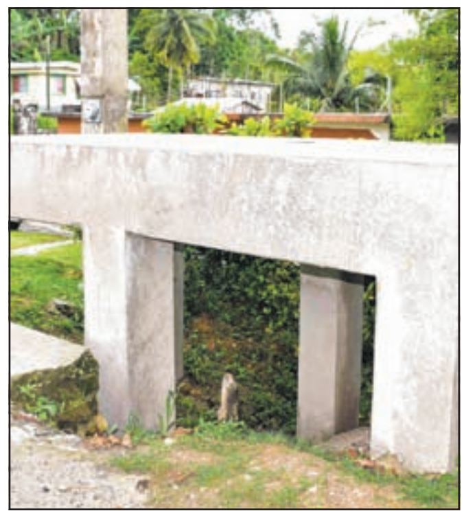
The base for a water catchment tank. Faced with severe droughts, many farmers in the Caribbean have found it necessary to set up catchment areas to harvest water whenever it rains. Caribbean Development Bank
