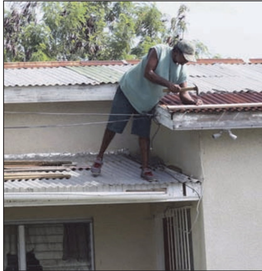
A homeowner makes last minute repairs to his roof in preparation for Hurricane Irma, in St. John's, Antigua and Barbuda, Tuesday, Sept. 5, 2017.
